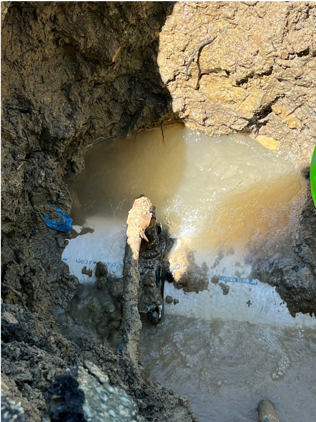
Attachment 1: Townwood Water Leak – Saddle Failure
